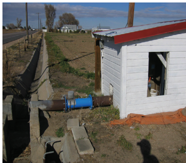
Installed flow meter
